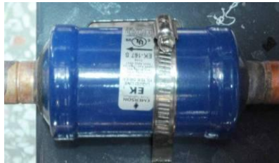
Picture 2-29: Drying Filter
