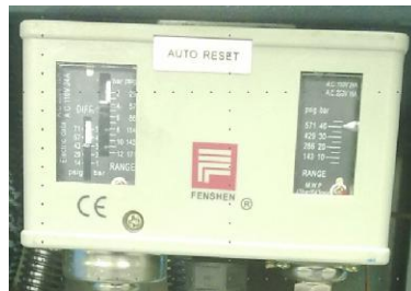
Picture 2-32: High and Low Pressure Controller
